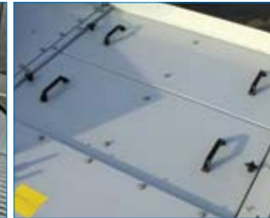
Distribution basin covers*
