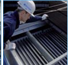
on site services
