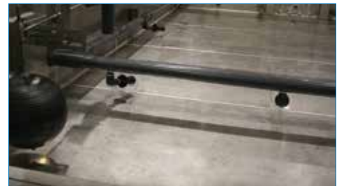
Cold Water Basin with Sweeper Piping
