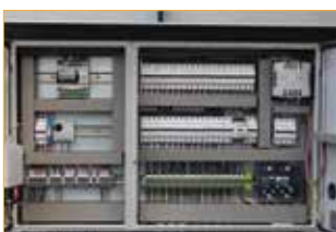
Integrated controls with separate control and power panels
