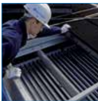
on site services
