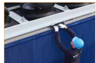
Critical components accessible from outside during operation
